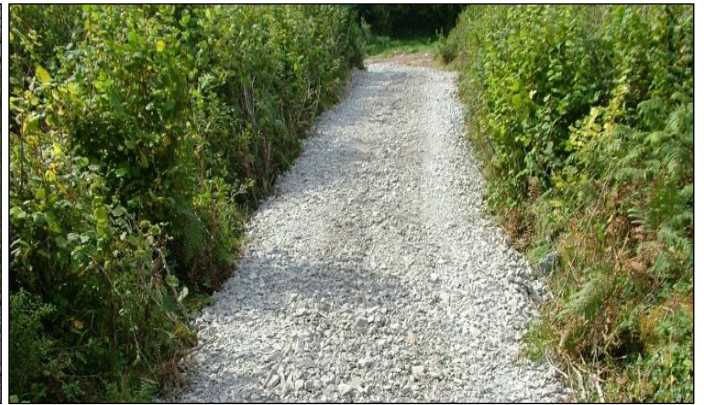
Excessive use of chip across full track width.
