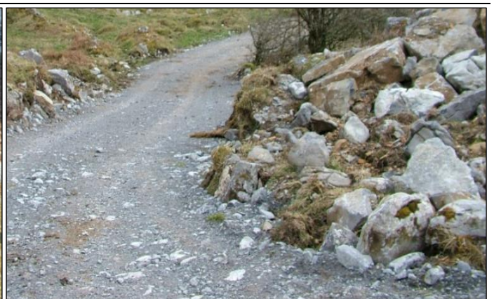
Excessive disturbance and excavation of bedrock.
